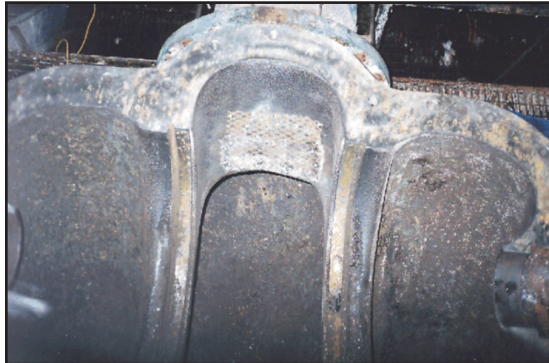
Damaged surfaces of pump
